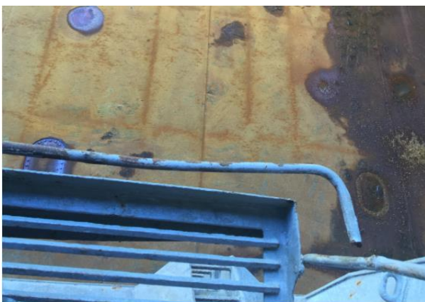
Figure 11: The damages at the second platform railing of the vertical ladder
